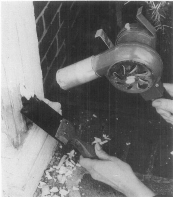
Fig. 14 The nozzle on the electric heat gun permits hot air to be aimed into cavities on solid decorative elements such as this applied column. After the paint has been sufficiently softened, it can be removed with a profiled scraper. Photo: Charles E. Fisher, III.
